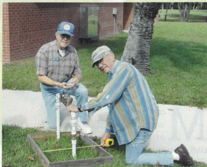
Paul Clark and Virgil Mashburn working with the maintenance department to repair some pipes.
