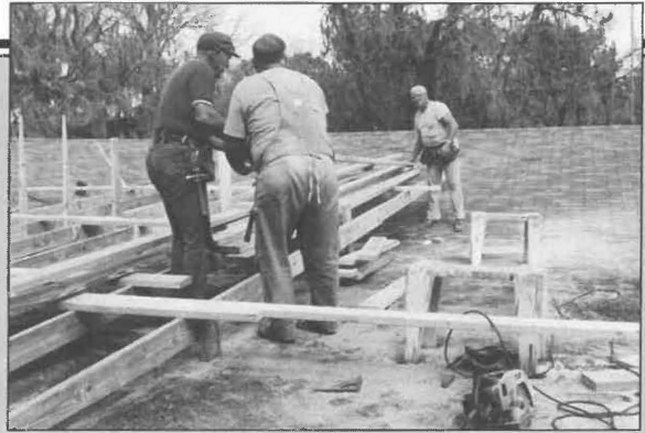
A flat portion of the Lewis Cottage roof was rebuilt and given a pitch to overcome a chronic leak.
