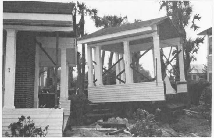
A small porch had to be removed and reattached after the house arrived at its destination.
