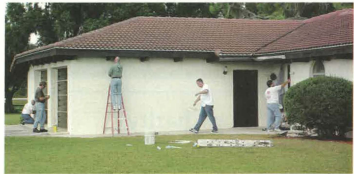
Another group jumps right in with taping the garage doors, trimming the roof line and rolling the side walls.
