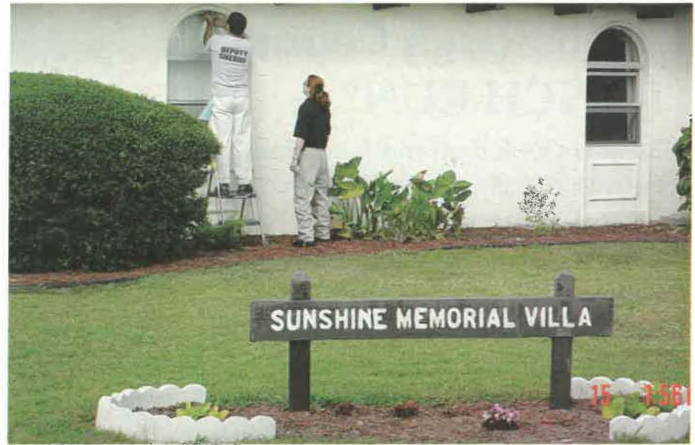
Taping out the windows on Sunshine Cottage at the Youth Villa is one of the first tasks of the day for a few members of the Hillsborough County Sheriffs Office training team.
