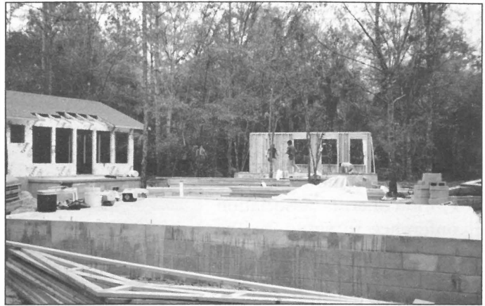
CARUTH CAMP — Construction was in the early stages when these photos of the cabins were taken in early January.
