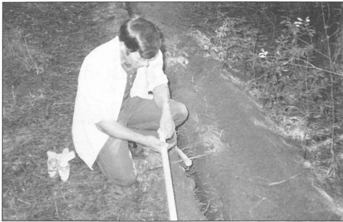
CARUTH CAMP — Being extremely careful to avoid areas of tree roots, Caruth Camp maintenance employee Larry Holbrook lays PVC pipe for waterlines in preparation for the Raymond and Myrtle Whitaker Campsite construction.
