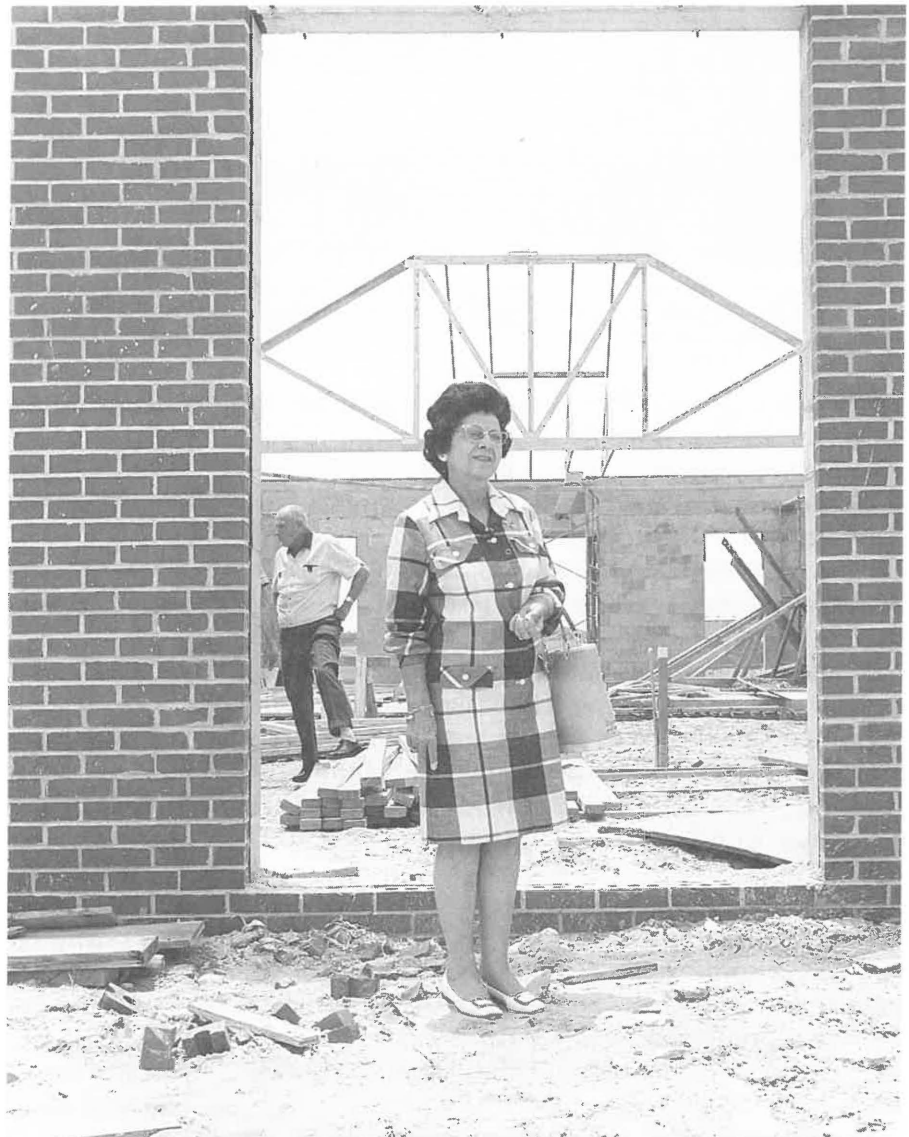
The Boys Ranch Chapel was under construction and Trustee Frances Diaz was on an inspection tour when this photo was taken in 1966.
