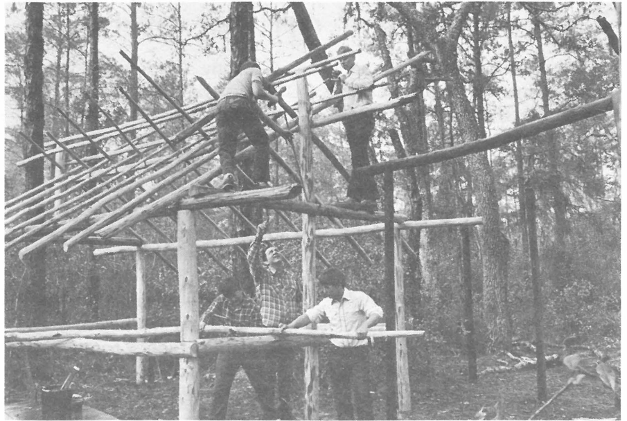
Peeled pine poles held together with wooden pegs will become a cooking shelter.
