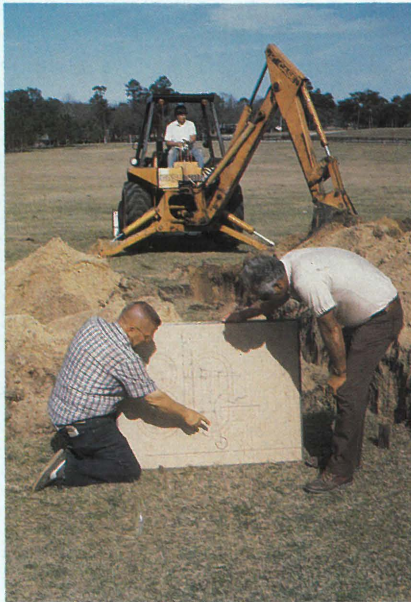
While foundation work was in progress for the 30-foot star, J.B. Brettingen (kneeling) explained his design to Kenny Gilley, Boys Ranch Supervisor of Maintenance.
