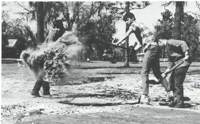
Rebuilding roads is one of the projects scheduled at the Boys Ranch for 1970 — but meanwhile there are many potholes to be filled after each heavy rain.
